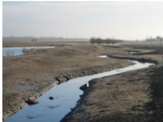
View of the Tullstorpsån stream area at Sånarp directly after the wetland construction. For the 2020 view, look at the frontpage. Photo: Johnny Carlsson
